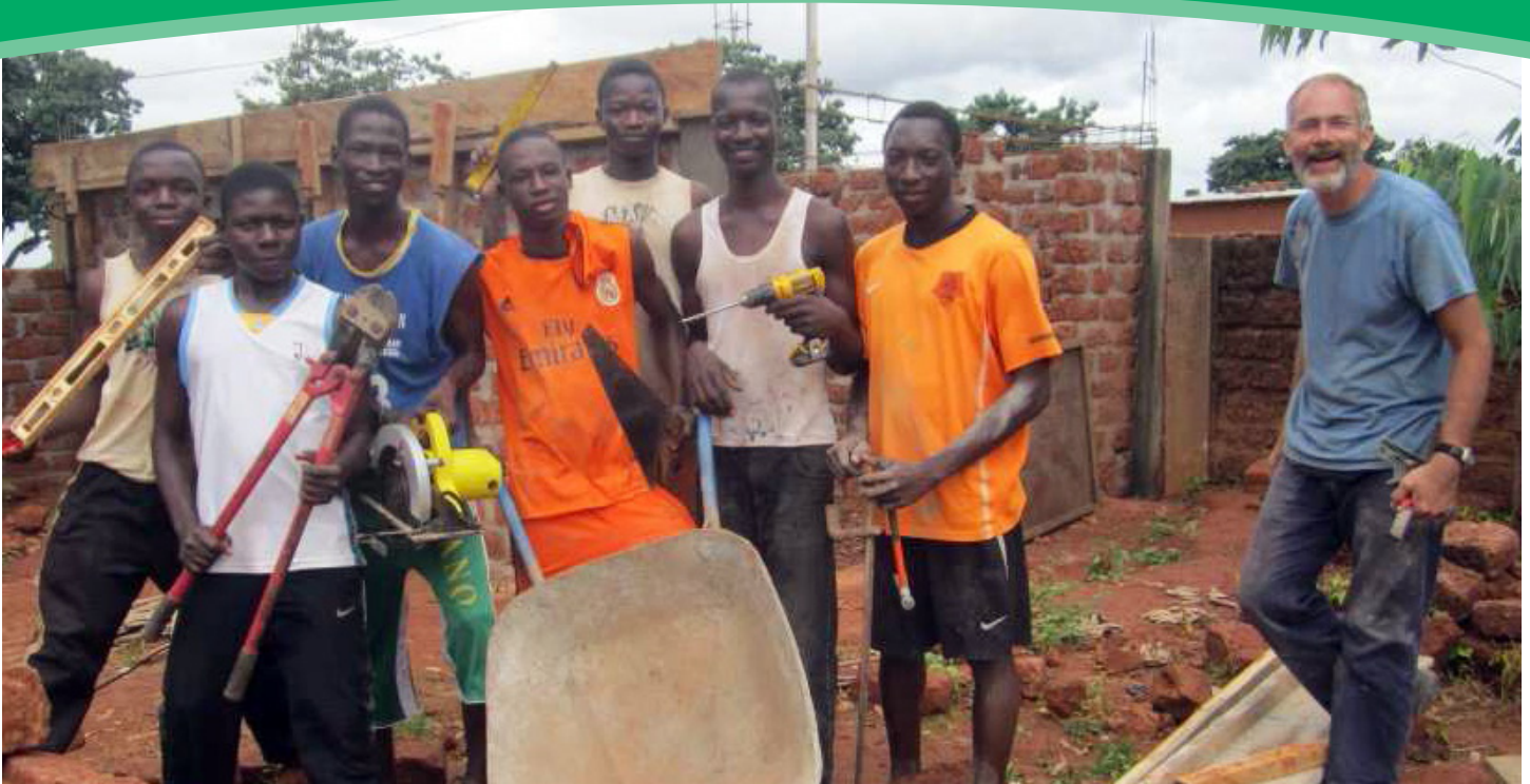
Local church youth in Burkina Faso helped build a welding workshop that will be a small business and a classroom to learn the trade.
